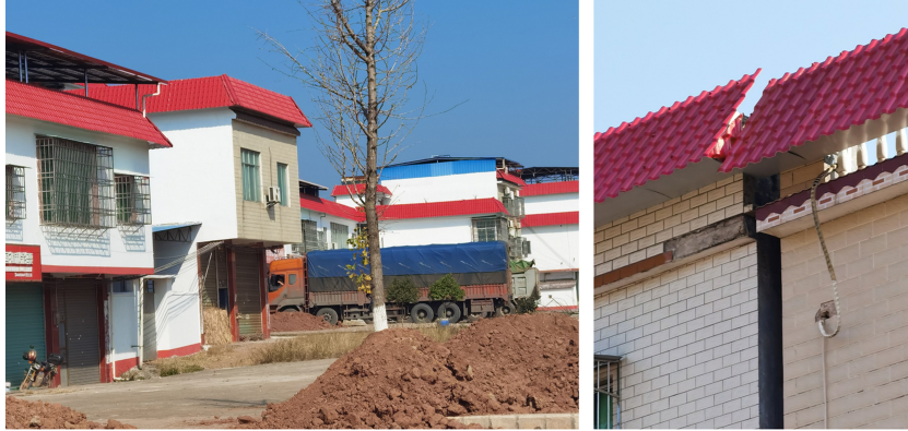
Figure 4 The lack of guidance in “flat-to-sloping” roof conversion practices does not yield satisfactory results in aesthetics and safety
