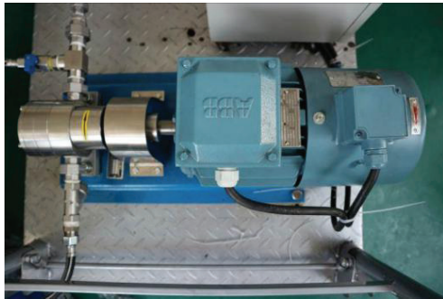
Figure 5 Gear metering pump and variable frequency motor
