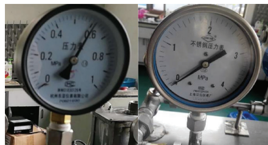
Figure 9 Pressure gauge of water and oil pipeline
