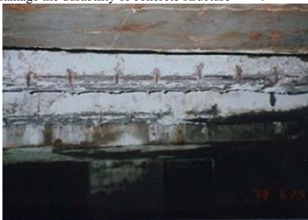
Figure 2 marine corrosion surface [41]
