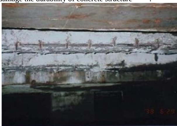
Figure 2 marine corrosion surface [41]
